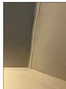
Tape joint(s) were peeling or damaged. This is not a typical sign of structural movement in most cases. This is usually a cosmetic defect caused by expansion and contraction due to change in temperature. Evaluate and repair. (Blue)
