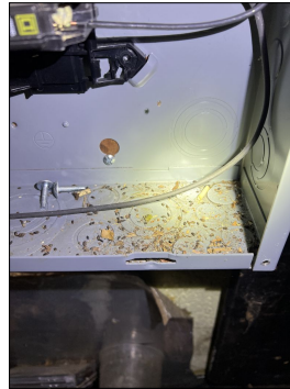
Rodent droppings or signs of rodents were observed in the breaker panel box at the time of inspection. Recommend having any access to the panel sealed to prevent intrusion of pests that can lead to damaged wiring. Evaluate and repair as needed. (Blue)
