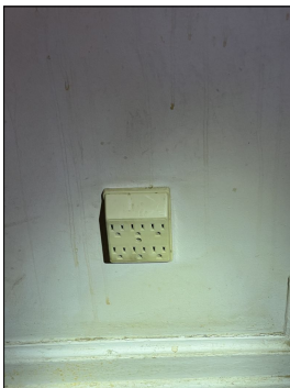
It is recommended to avoid use of multiplier outlet plug ins(converts 2 into 6 outlets). Unable to test outlet and/or verify if the outlet is GFCI protected(only in locations where needed). Recommend removing and replacing as needed. (Blue)
