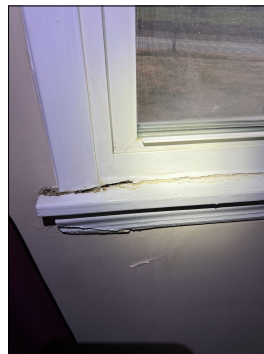
Water penetration observed at the wall below the window and damage consistent with water at window trim. Unable to determine if the windows were properly sealed. Recommend sealing and maintaining the seal. Recommend review of the window to determine if the installation is correct. Evaluate and repair or replace as needed. (Red)
