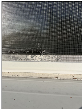
Damaged window screens. Repair or replace as needed. (Blue) Location: Review all windows
