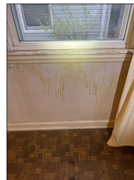
Discoloration or defects at walls. Normal moisture levels at time of inspection. Location: Main floor Bedroom 2
