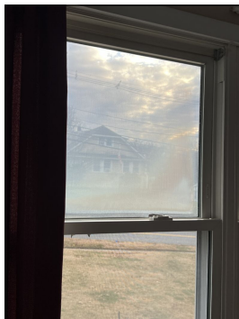
Condensation, staining or fogged glass at double pane windows typically indicates a broken seal between the panes. Repair or replace as needed. (Blue) Location: Review all windows
