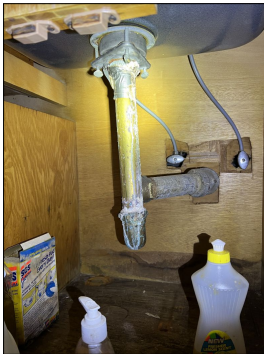
Moderate corrosion at drain lines. Leaking may occur if not repaired. Evaluate. Repair or replace as needed. (Purple)
