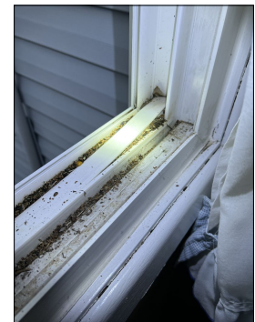
Damaged window components observed. It appears as if nesting occurred in the window. Recommend sealing any gaps or openings around the exterior of the home. Evaluate, treat and repair as needed. (Blue)
