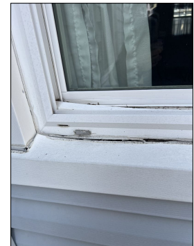
Caulk was damaged at time of inspection. Maintain caulk at exterior window trim, to help prevent intrusion of water, pests/rodents and/or WDI. Evaluate, maintain and/or repair as needed. (Blue)
