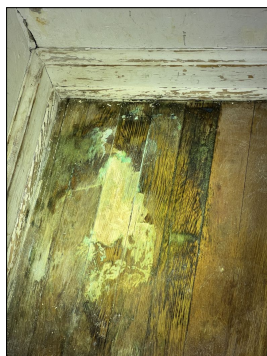
Discoloration observed at the floor boards. Areas of the hardwood floor appeared to be damaged and appears to be cosmetic. Evaluate and replace as needed. (Purple)
