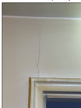
Minor to moderate defects or damage to walls; cracking plaster or drywall, tape joints peeling and/or popping nails, damaged drywall. Recommend adding a door stop behind the door to prevent the hardware from hitting the wall. Repair as needed. (Blue)
