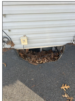
The window well cover was missing, recommend installing window well cover to prevent water intrusion, foliage and/or vegetation growth. Evaluate and replace as needed. (Purple)
