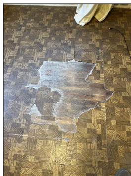
Laminate and/or vinyl floors were Damaged. Repairs should be made to prevent slips, trips or falls. Evaluate and repair as needed. (Blue)
