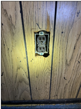
Missing outlet/switch cover plate(s). Replace for safety. (Red)
