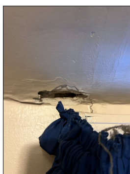
Openings observed in the drywall. Not a major concern, typically. Unless water intrusion or other defects couple with the damages. No signs of other defects. Recommend repairs. Evaluate and repair as needed. (Blue)
