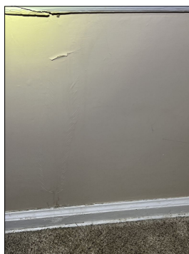
Signs of previous water damage or leaks at walls. Walls were dry at the time of inspection. Recommend determining if a moisture source is still present and repair as needed. Evaluate and repair as needed. (Purple)
